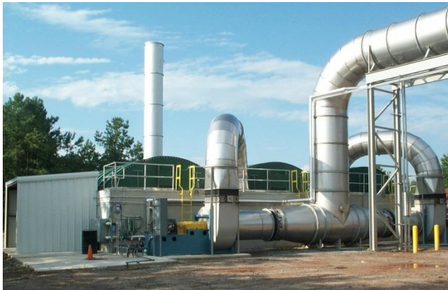
86,000-CFM high-capacity biofilter system for the treatment of odors and VOCs at an industrial facility
