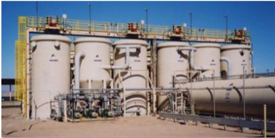
Figure 3: Envirogen FBR for Perchlorate Removal
